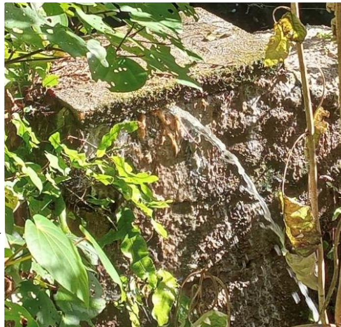
The 2022 leak at the north bank
